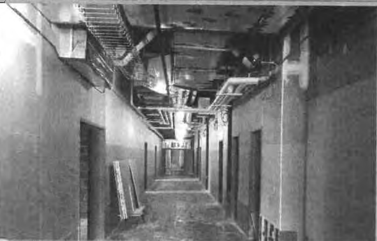
Corridor - MEP (Mechanical/HVAC, Electrical, Plumbing) _ 10.01.2018
